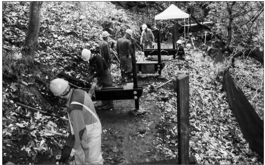
The Twin Oaks Construction crew in action, building boardwalks and a bridge in Oaks Bottom Wildlife Refuge and Marquam Park in Portland.
